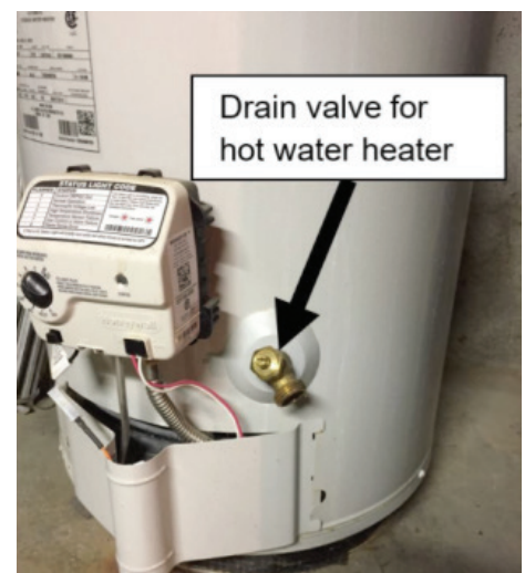
FIGURE 6 Water heater with drain valve
