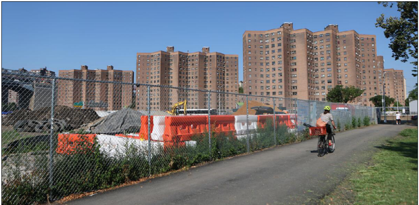
Some co-ops will be protected from storm surge-based flooding by neighborhood-scale projects like the East Side Coastal Resiliency Project (under construction here in this photo). However, this project will not protect from rain-based flooding. (Source: EDF)
